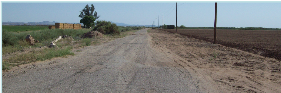
Example of a roadway with very poor pavement condition
